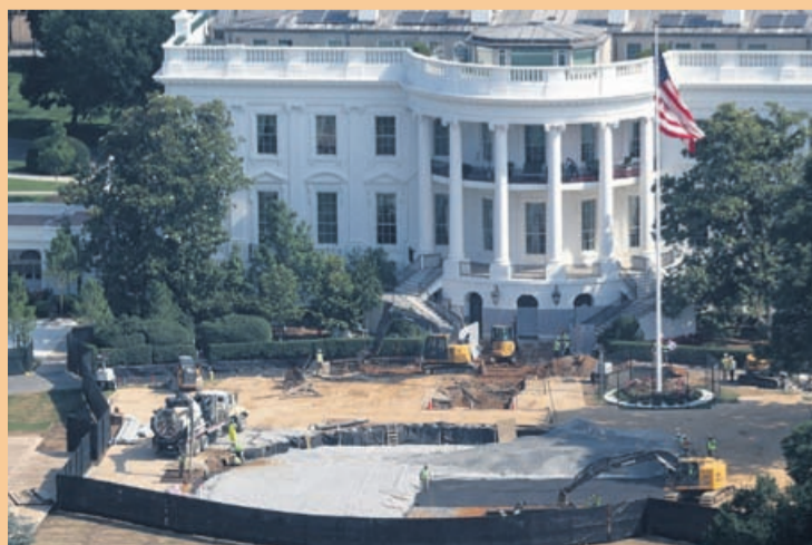
Construction of a new helipad on the South Lawn of the White House continues on July 01, 2026 in Washington, DC.
