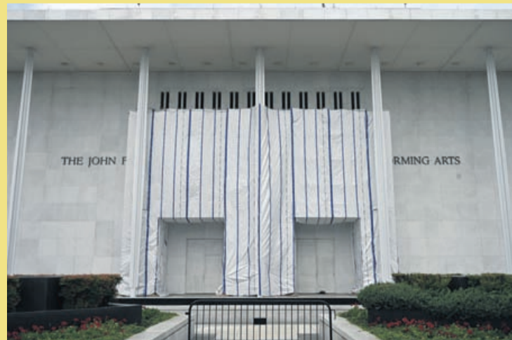
A tarp covers the facade of the John F. Kennedy Memorial Center for the Performing Arts in Washington, D.C., on June 14, 2026.
