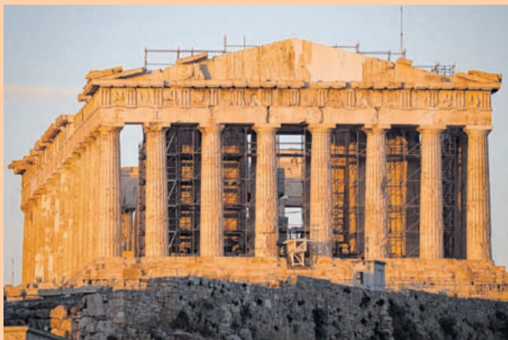
This photograph shows the ancient Parthenon temple atop the Acropolis, free of external scaffolding after renovation work, in Athens on June 18, 2026.
