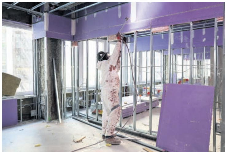
A worker paints at 77 Water Street, a former office building being transformed into luxury rental apartments in the Financial District of New York, on April 10, 2026.
