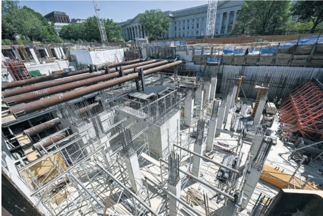
A view of the construction site of U.S. President Donald Trump's proposed ballroom as he speaks to the press at the White House in Washington, DC, on May 19, 2026.
