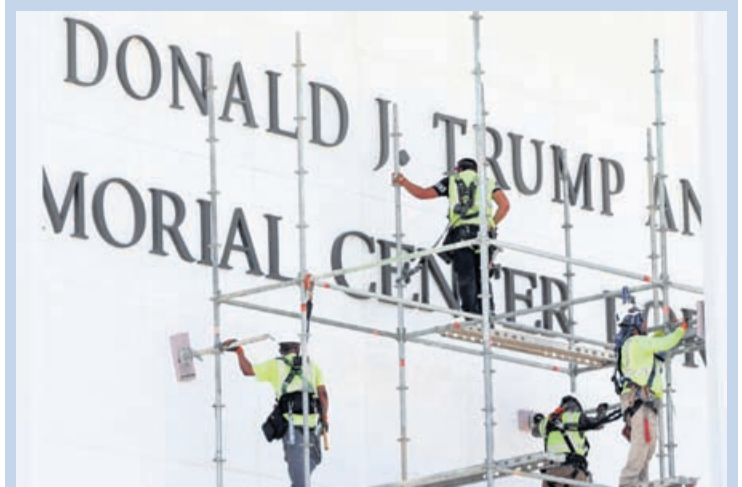
Workers stand on scaffolding near the signage for the Donald J. Trump and John F. Kennedy Memorial Center for the Performing Arts in Washington, DC, on June 12, 2026.
