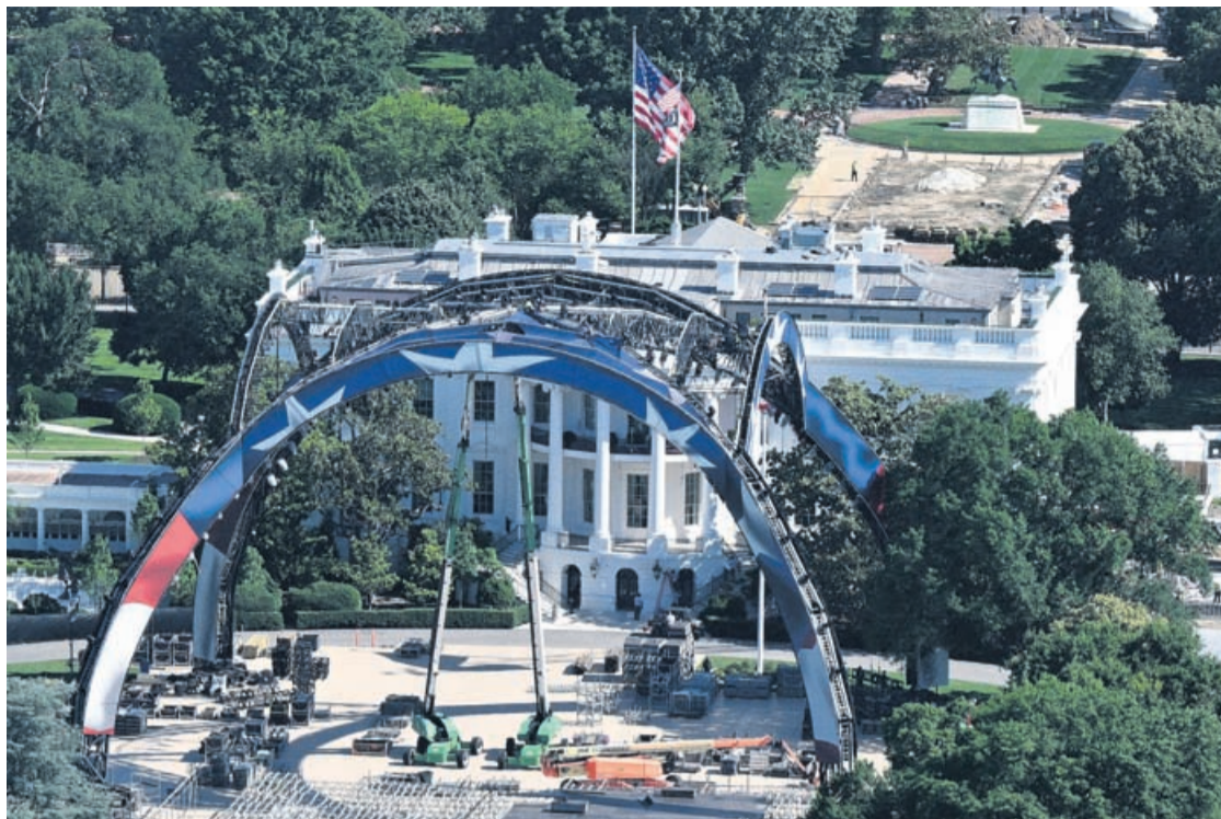
Cranes work on the construction of a structure on the South Lawn of the White House in Washington, DC, on May 29, 2026, for the upcoming UFC fight that US President Donald Trump will host as part of the 250th anniversary of the United States.
