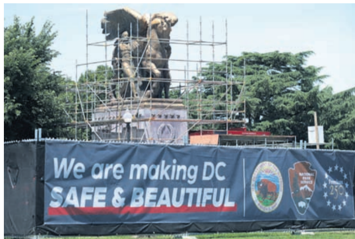
Workers build a scaffolding around one of the two The Arts of Peace statues near Lincoln Memorial for a restoration project on May 29, 2026 in Washington, DC.
