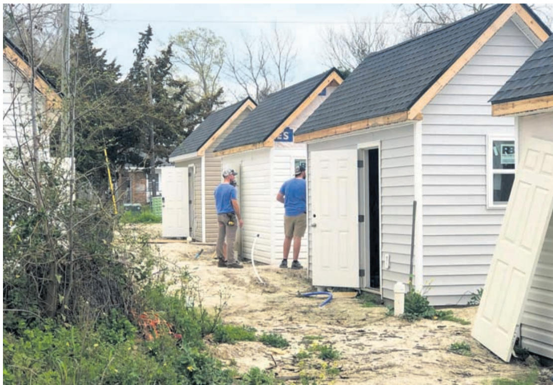
Contractors build tiny homes in Little River for Veterans Welcome Home and Resource Center.
