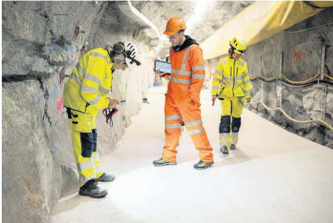
ETH Zurich Master students Alba Zappone, Alessandro Profeta and ETH Zurich doctoral student Lu Tian examine the cracks in the BedrettoLab tunnel, a unique underground research facility operated by the Federal Institute of Technology Zurich (ETH Zurich) located 1500m beneath the Swiss Alps within a 5.2 km tunnel near Bedretto, on April 29, 2026.
