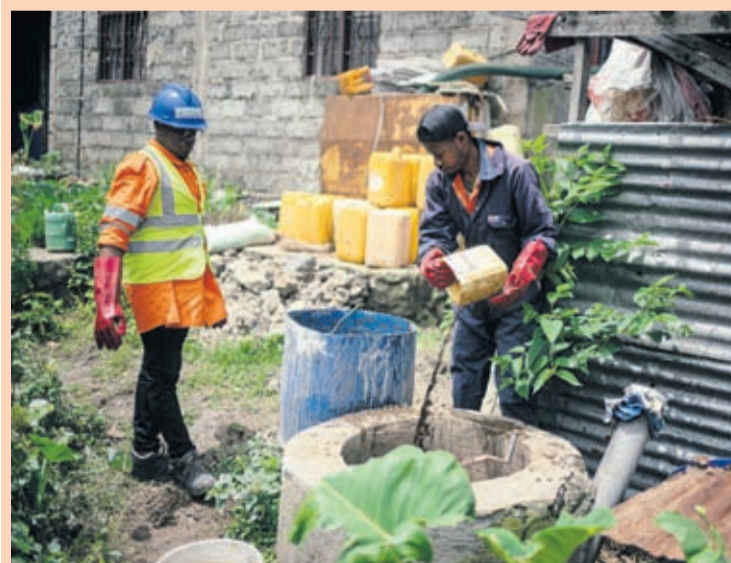
Victoire Materanya (L), co-founder of Umoja, watches as a worker mixes waste from a duck enclosure to put in the digester in order to produce clean energy in Goma on April 20, 2026.
