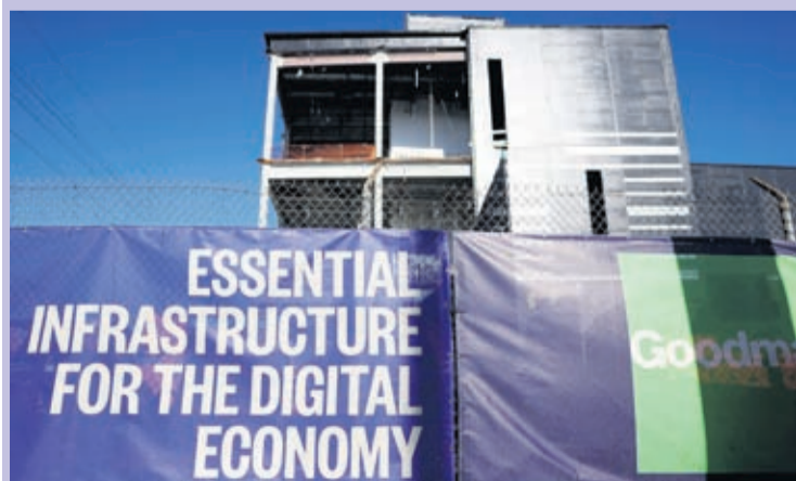
A view of a 49.5 megawatt three-level data center under construction on April 14, 2026 in Vernon, California.
