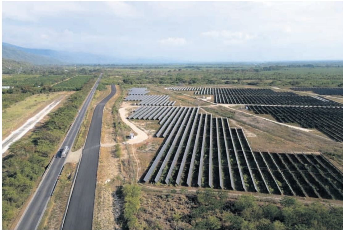
Aerial view of the solar park in Zona Bananera, Prado Sevilla, Magdalena department, Colombia on April 17, 2026.
