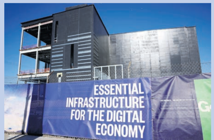
A view of a 49.5 megawatt three-level data center under construction on April 14, 2026 in Vernon, California.
