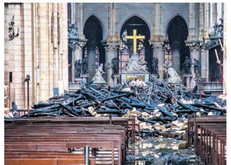
A hole is seen in the dome inside Notre Dame cathedral after the fire in Paris, Tuesday, April 16, 2019.
